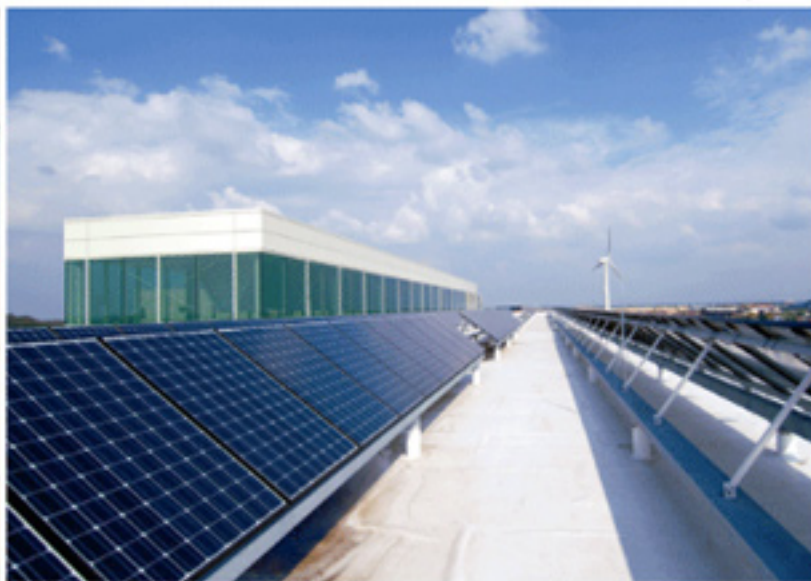
These are roof-mounted photovoltaic fixed arrays, with the 200 kW wind turbine in the background. The arrays are connected to a series of dc-ac converters. Photo: Lucie Marusin
